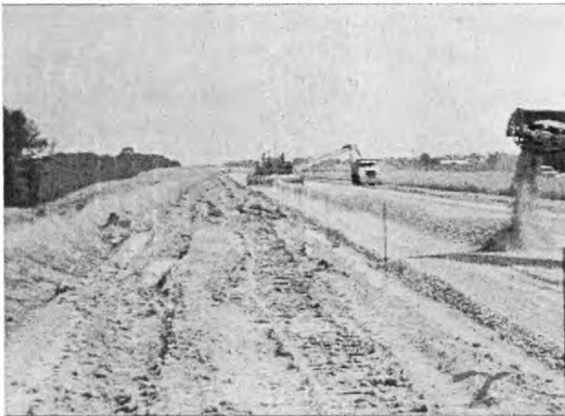
Figure 40. Placing trimmed aggregate back in to the haul trucks for re-use at other location
