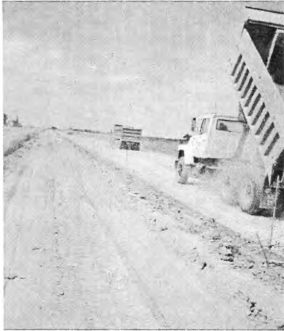
Figure 34. Unstable shoulder under loaded trucks placing aggregate
