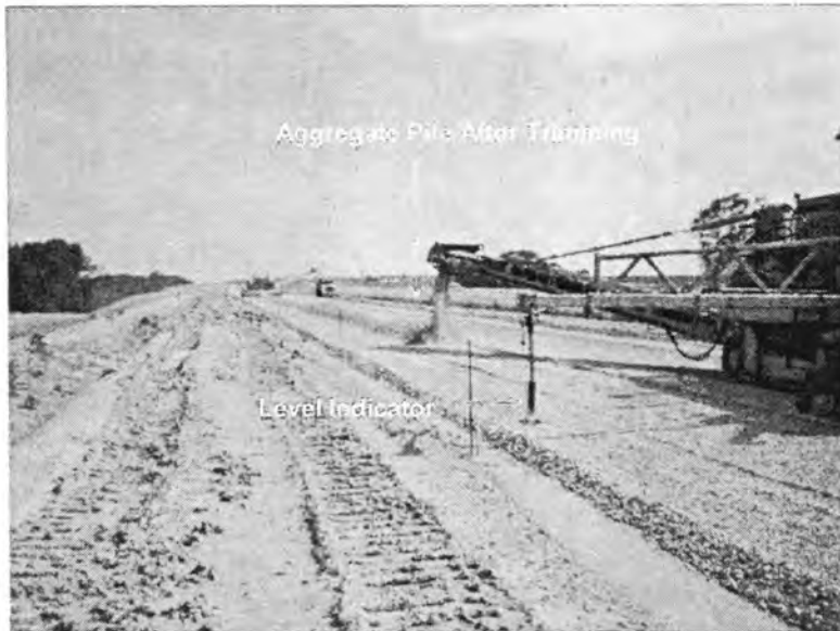
Figure 39 Final trimming of base, level indicator attached to trimmer, and aggregate pile formed after trimming
