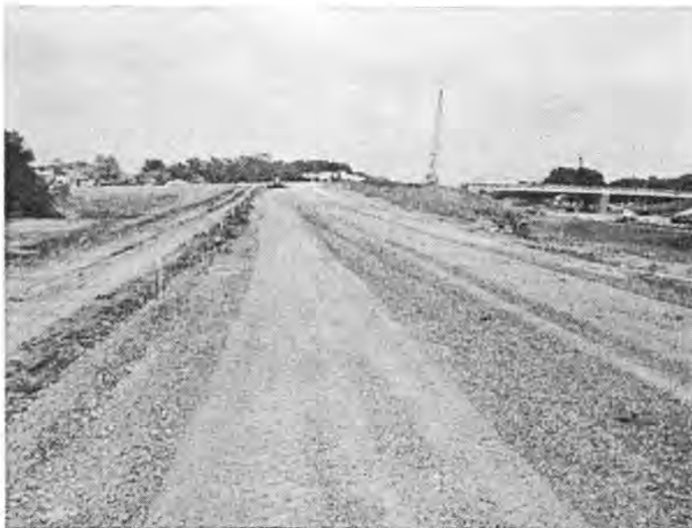
Figure 56. Photograph of the modified subbase layer during construction at 35 th street test section
