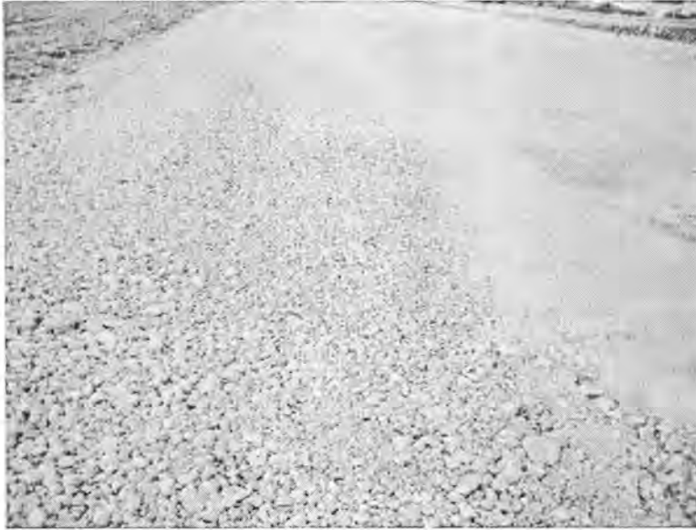
Figure 58. Picture showing segregation in fines on the final base layer
