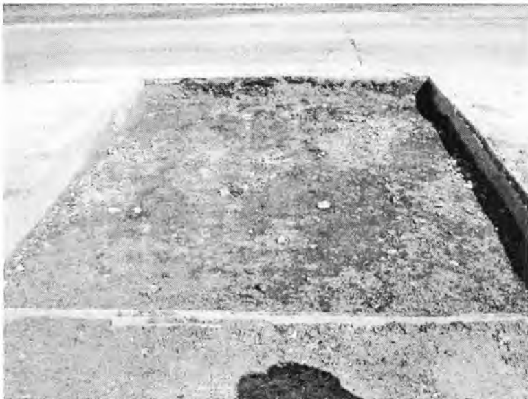
Figure 73. Test section used for DCP testing to investigate the spatial variability US Hwy 30
